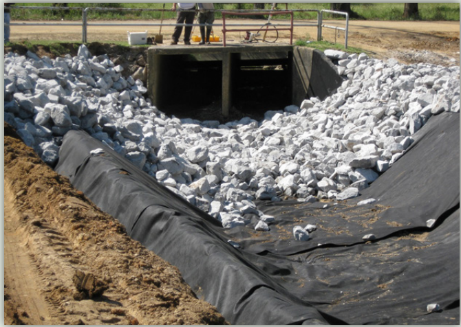
Additional drainage improvement projects along Town Creek should remain a priority for the City of McComb.
