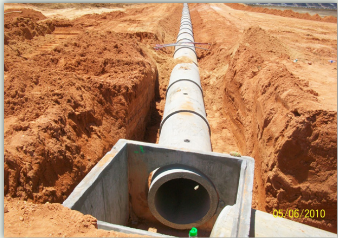
Improvements to the existing sewage collection system will reduce McComb’s ongoing problems with inflow and infiltration.
