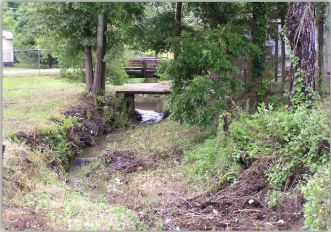
Storm drainage system deficiencies remain city-wide, and cause flooding on residential properties, and inhibit investment in valuable property along Town Creek in the Canadian Railroad rail yards.
